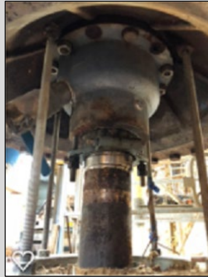
Before: Leaking blow tank bottom entry vertical agitator
