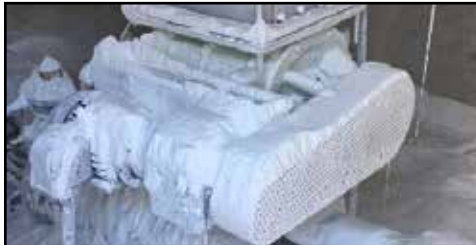
Rotary valves are prone to expensive and unsafe leakage due to ineffective shaft seals
